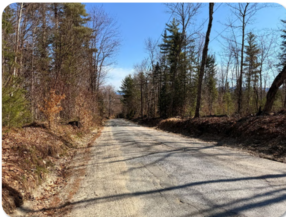
Photo 4: View of roadway condition looking north.
